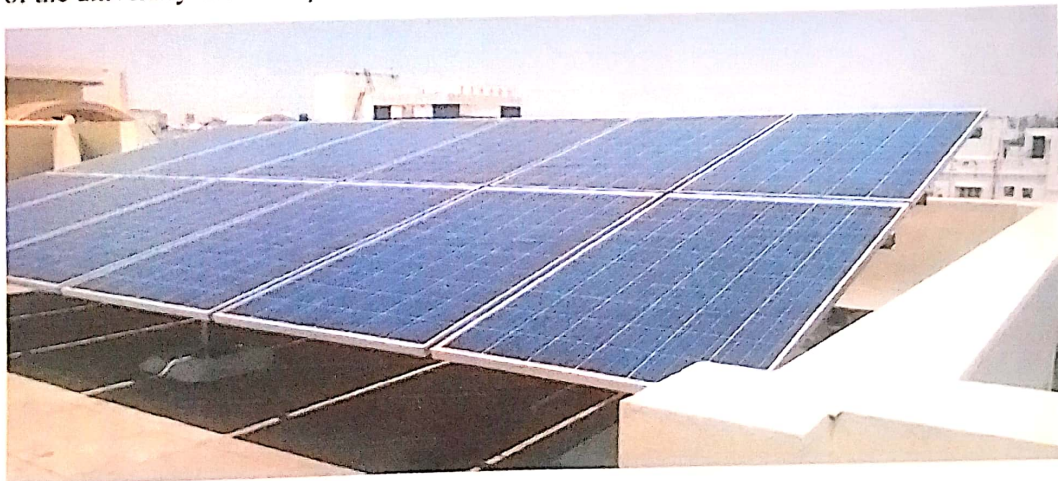
5KW on GRIDTIE SOLAR SYSTEM
